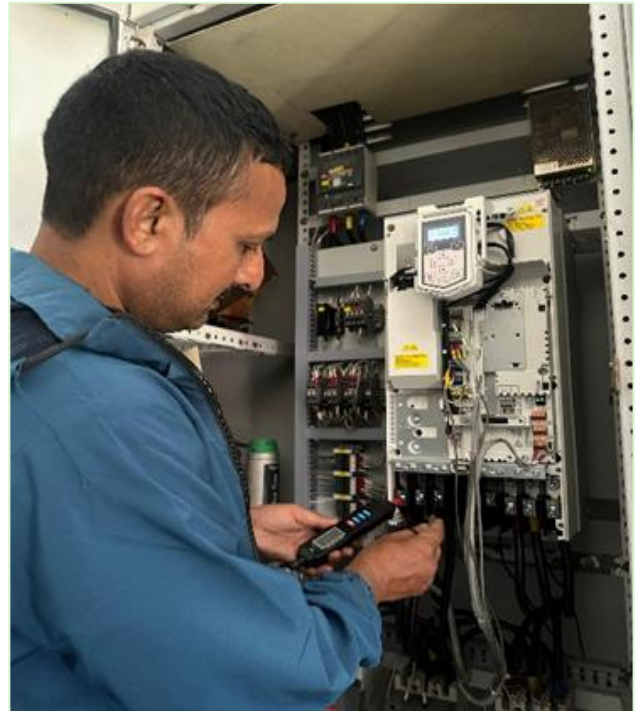
Fig: Installation of VFD for Backwash Pump system
