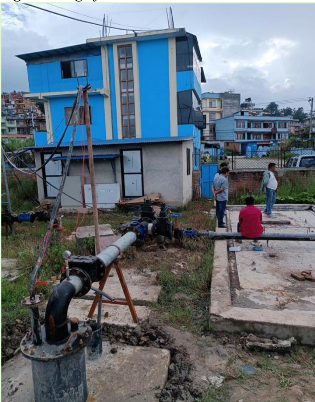
Fig: New sumpwell brought into operation at Kirtipur SRT
