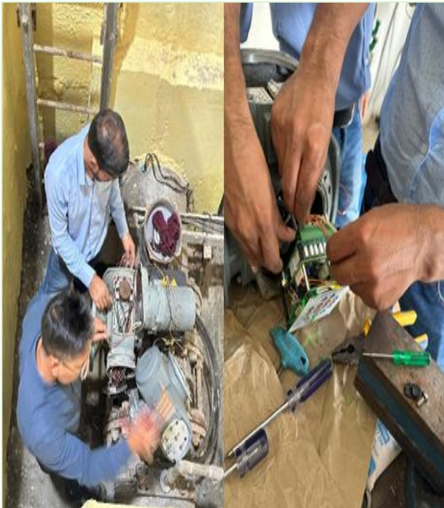
Fig: Maintenance of Rapid Sand filter actuator system
