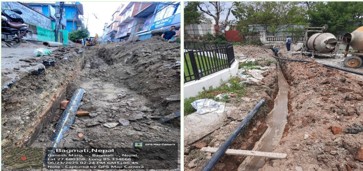
Fig: 100mm dia. Pipeline Improvement at Ganesh Marg ( To improve the distribution line, Reduce the pipeline leakage & new water line connection work has been completed)
