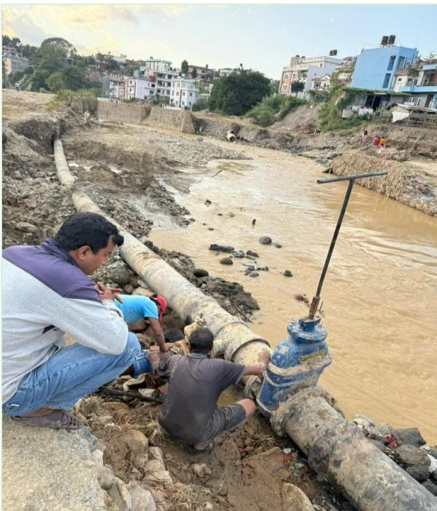
Fig: 16" valve and pipeline rehabilitation work damaged by flood at Kantipur colony
