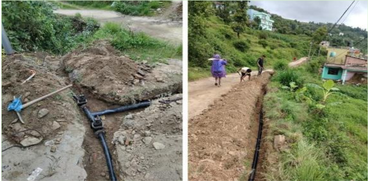
Fig: Water supply pipeline ( 4" and 2" dia. HDPE) extension work completed at Brahmayani, Bhane, Bhaktapur increasing the service area of the KUKL.
